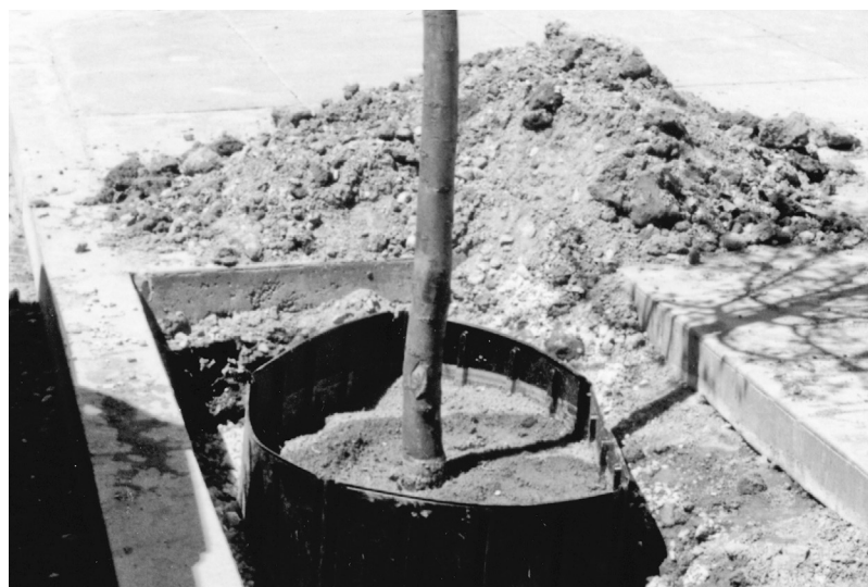
In the case of this newly planted tree, the strategy is to place backfill outside the barrier that will favor root growth after it is forced downward by the barrier.
