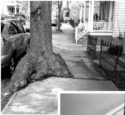
The problem in this case is made worse by a cut of the trunk flare, risking stability and health of the tree.
