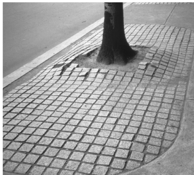
One of many solutions — loose-laid pavers that can be removed as the tree expands.
