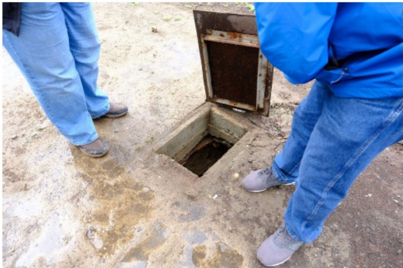
Underground Collection Tank
