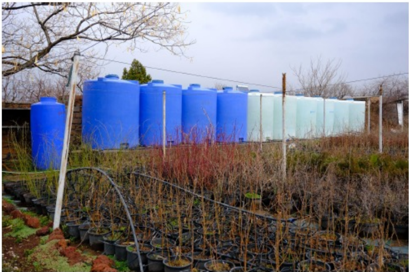
5000 L Storage Tanks
